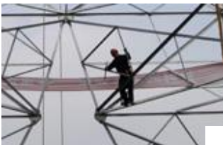
Labourers repair electrical pylons on the outskirts of Pingxiang, China (Photo: Reuters)
